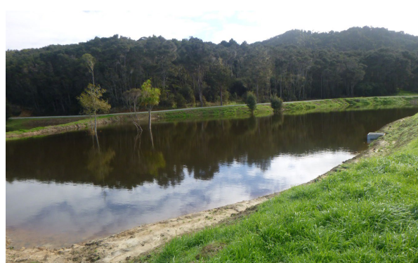
Lower valley weir. Note water control structure, good vegetation cover and well-constructed access road.
